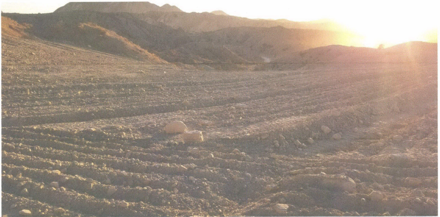
Photo 7: View facing south after top soil added, graded, and furrowed for runoff control (December 2020)
